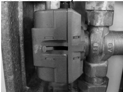
Suction of rain water from collection tank EP
